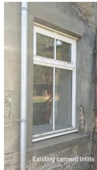
Existing cement infills
