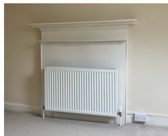
1 of 2no. existing fireplaces at first floor blocked, to be reinstated as part of the works
