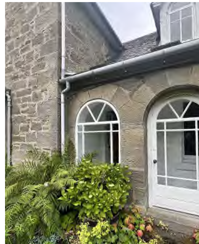
South Elevation showing poor quality UPVC rainwater goods and enclosed loggia window and doors, each to be replaced.
